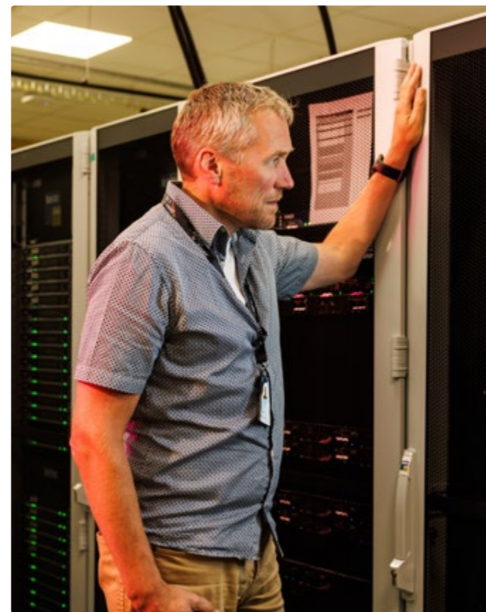
+ Egil Maurtvedt in the server room at Nittedal Teleport outside Oslo. Photo: Kilian Munch
